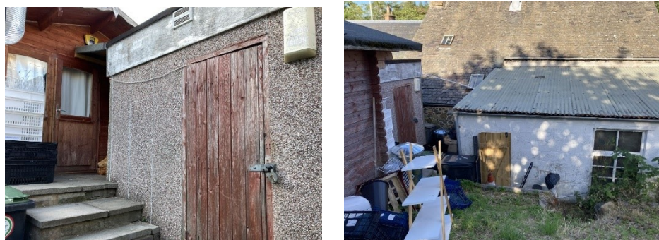
Challenging back yard of shop/ dangerous steps / poor buildings
